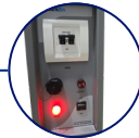
MCB and Ethernet Port, Power and Alarm Control, Main Power Switch, Battery Control Switch, Mains Indicator LED, and Alarm System Buzzer.
